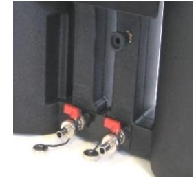
Service drain for draining during maintenance activities
